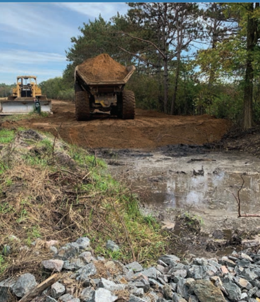
Removing a well and filling a large drainage ditch helped return flow to a nearly 1-mile headwater reach.
